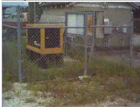
732-315 90 Gal. Diesel Fuel
