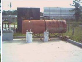
S736-02A 465 Gal. Used Transformer Oil
