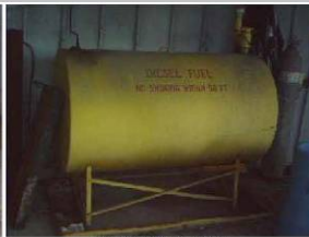
738-32A 260 Gal. Diesel Fuel
