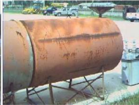
S736-01A 465 Gal. Used Transformer Oil
