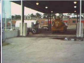
913-LJL 10300 Gal. Containment Volume
