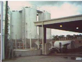
S362-06A (left tank) 20000 Gal., Used Oil
