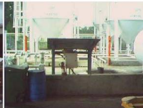
S362-07A (back right tank) 20000 Gal., Used Oil
