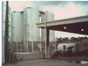
S362-05A (middle tank) 20000 Gal., Used Oil
