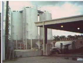
S362-06A (right tank) 20000 Gal., Used Oil
