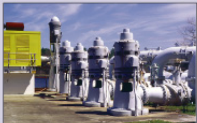
Public supply water intake, Bay County, Florida
