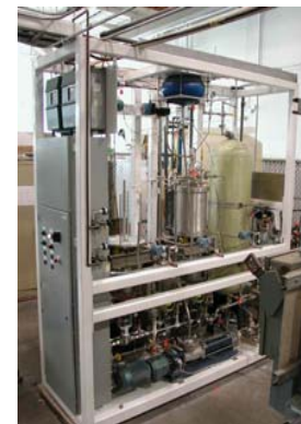
Heavy Metals Removal
